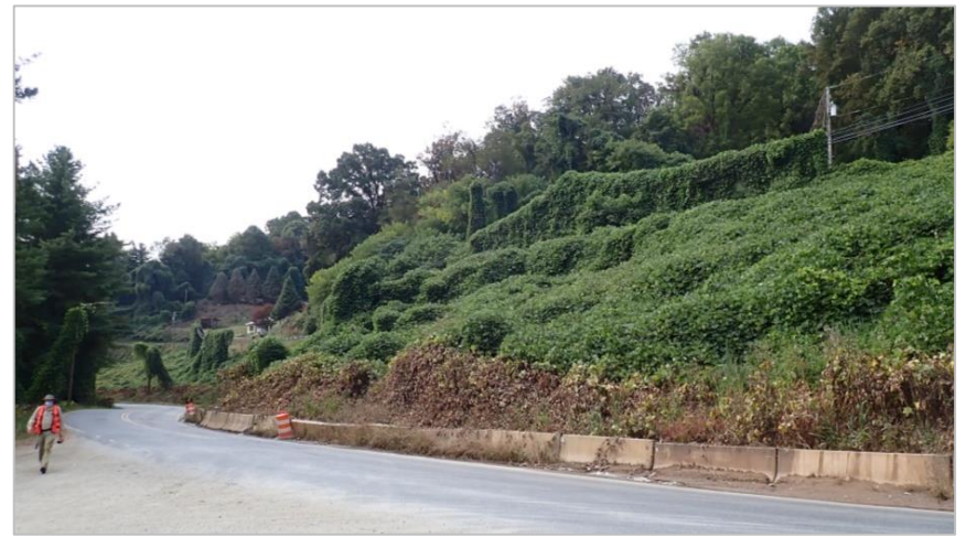
Figure 7A. Location A on map. Concrete median barriers at the toe of slope failure impinging on Chipper Curve Road. View looking NW. 10/08/2020 NCGS photo.
