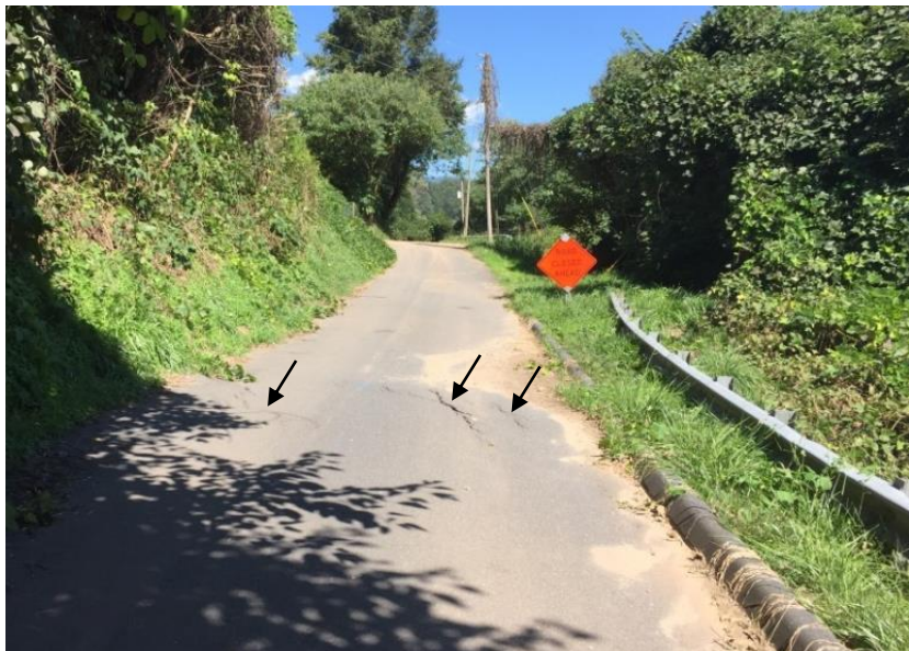
Figure 6C. Location C on map. Arrows point to ground ruptures in Allen Street pavement. Inferred movement direction toward the SE. View looking NE. 10/01/2020 NCGS photo.
