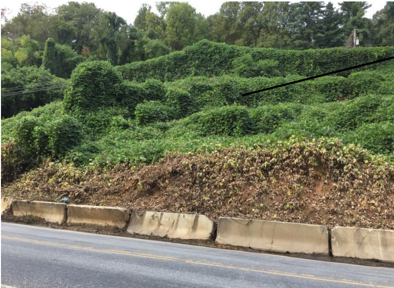
Figure 7C. Location C on map. Concrete median barriers at the toe of slope failure impinging on Chipper Curve Road in foreground. Leader line shows location of slide scarp in Fig. 7B right. View looking NW. 10/08/2020 NCGS photo.
