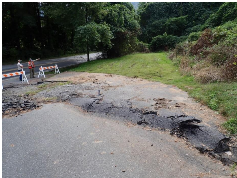
Figure 5C. Location C on map. Bulge in pavement from slide movement, Bryson Park entrance road. Ground bulging and wet ground was observed in the grassed area of the Park in the background. View looking southwest 10/08/2020 NCGS photo.
