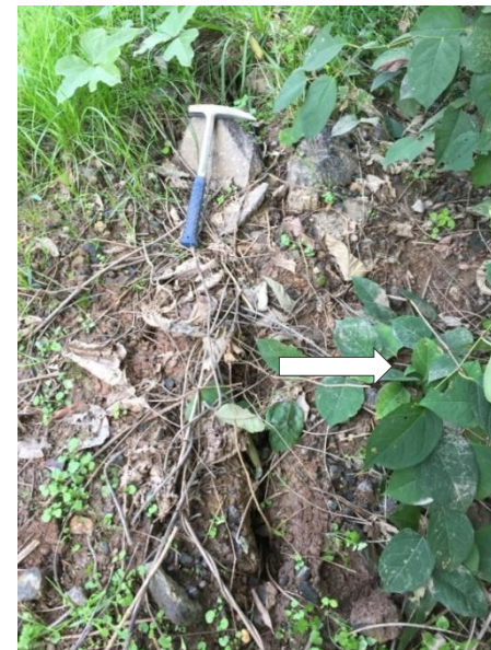
Figure 6B. Location B on map. Segment of ~30-ft long ground rupture in soil approximately 15 ft. SE of, and parallel to Allen Street. Arrow shows slope movement toward the SE. Hammer handle is ~14in long. View looking NE. 10/08/2020 NCGS photo.
