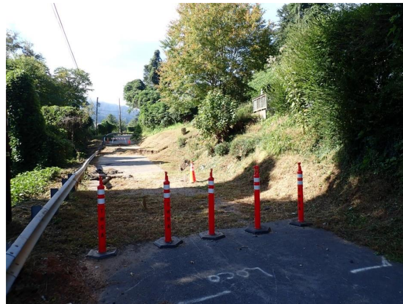
Figure 5A. Location A on map. Photograph showing down-dropped section of Allen Street. View looking southwest. 10/08/2020 NCGS photo.
