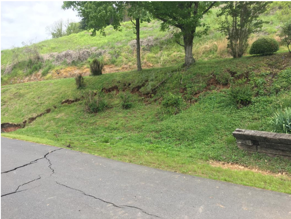
Photo 5: Extension of tension cracking up adjacent slope at 527 Allen Street. Photo dated 05/06/2020.
