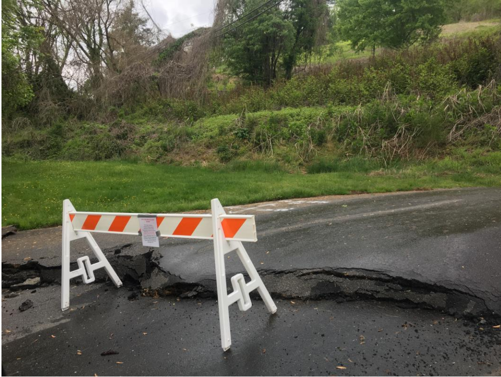
Photo 8: Slope Failure Area observed at Bryson Park entrance, facing west. Photo dated 05/06/2020.
