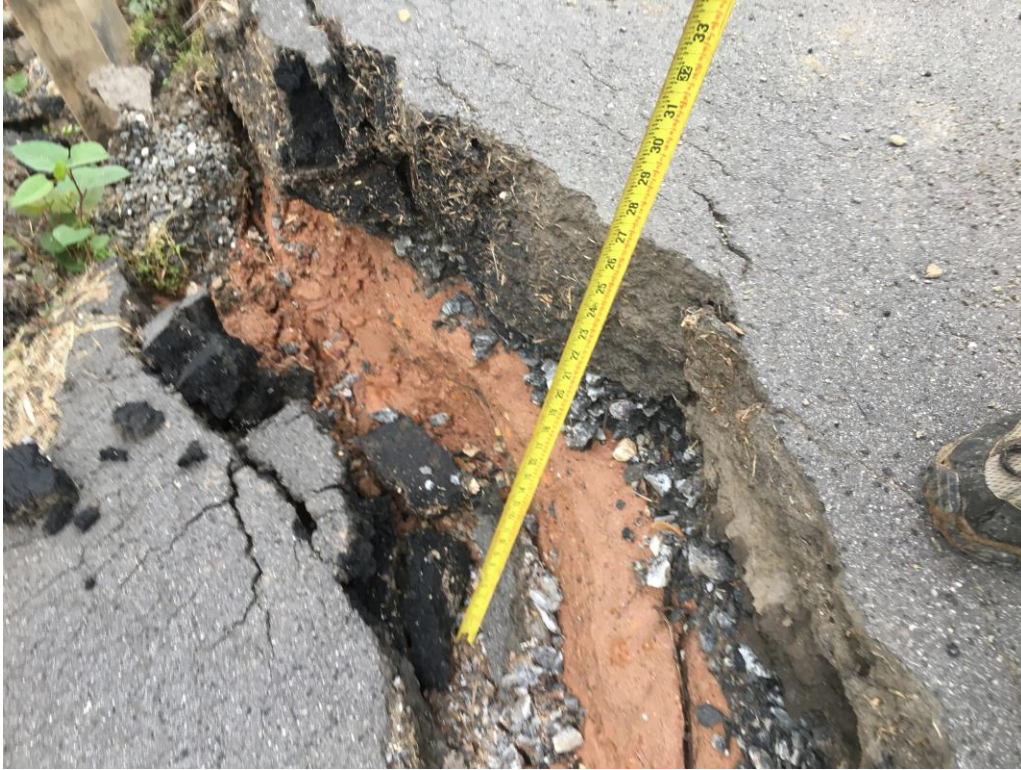
Photo 4: Approx. 2 feet vertical scarp on south edge of failure at Allen Street. Photo dated 05/06/2020.
