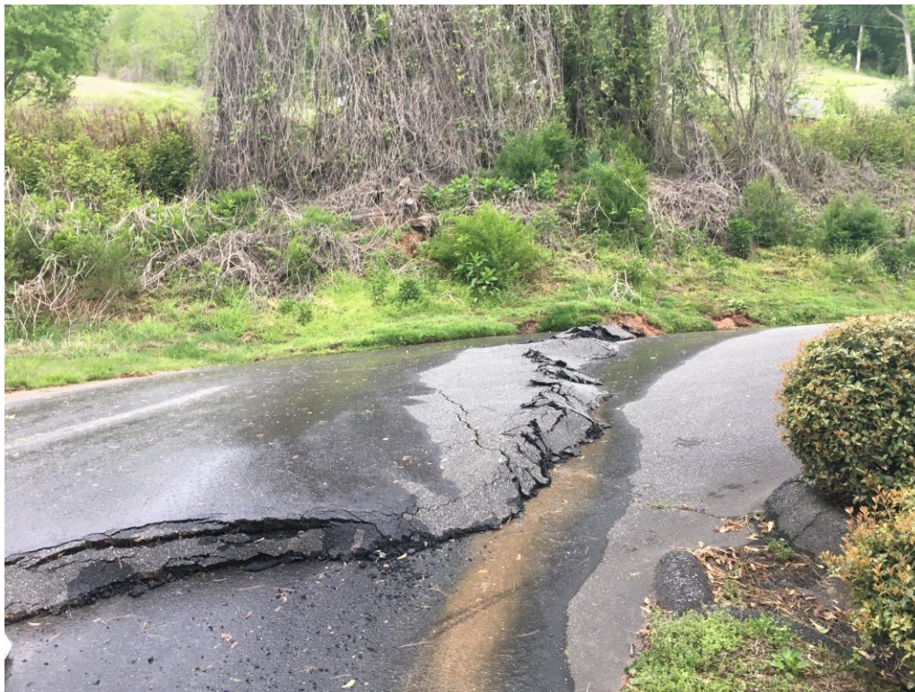
Photo 7: Slope Failure Area observed at Bryson Park entrance, facing west. Photo dated 05/06/2020.
