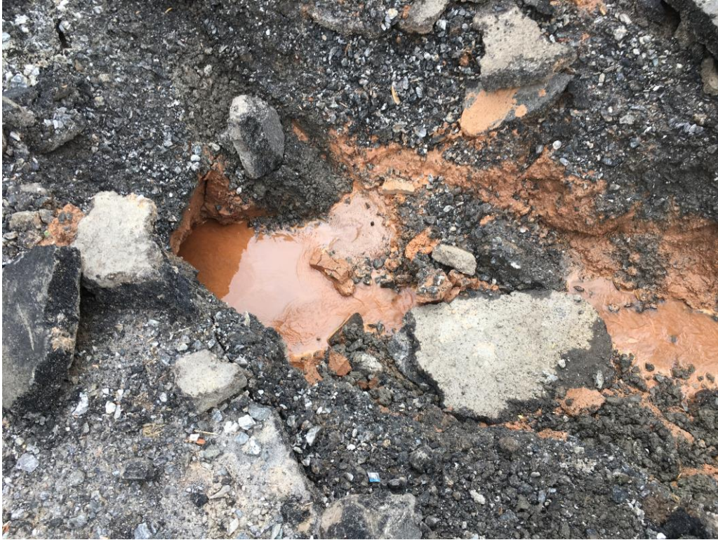
Photo 6: Water flowing near north end of failure within Allen Street. Photo dated 05/06/2020.
