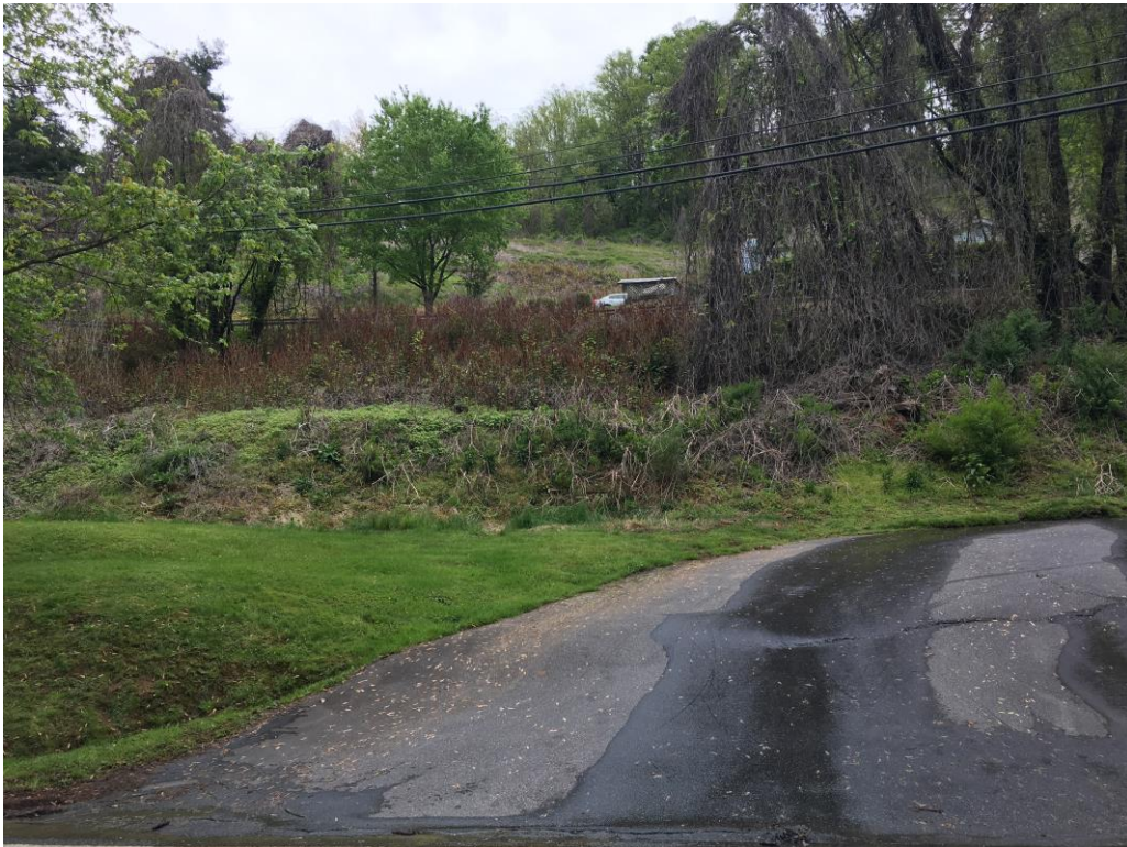
Photo 2: Slope Failure Area observed from Chipper Curve Road, facing west. Photo dated 04/30/2020.
