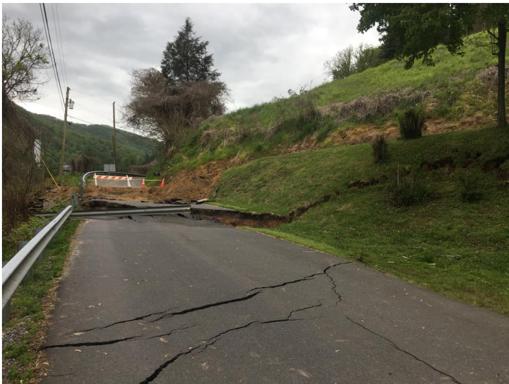
Photo 3: Slope Failure Area observed within Allen Street, facing south. Photo dated 05/06/2020.
