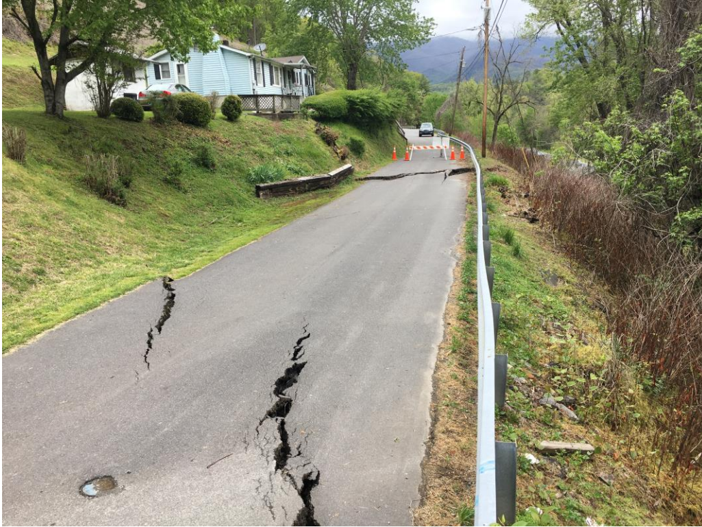
Photo 1: Slope Failure Area observed within Allen Street, facing north. Photo dated 04/30/2020.
