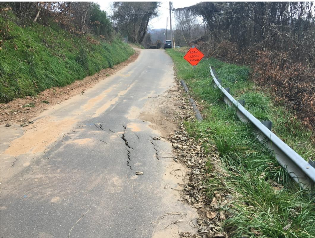
Photo 2: Tension cracking within Allen Street, approx. 180 feet SW of Bobwhite Lane, vicinity of B-14, photo facing northeast. Photo dated 11/25/2020.
