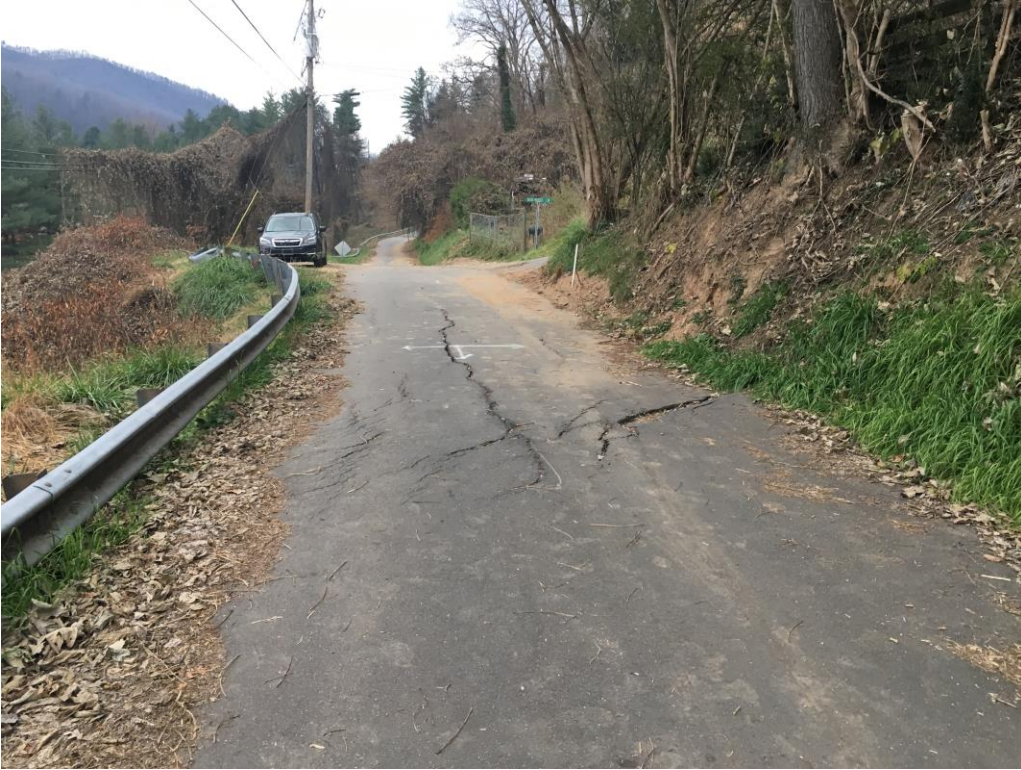
Photo 1: Tension cracking within Allen Street, approx. 30 feet NE of Bobwhite Lane, vicinity of B-11, photo facing southwest. Photo dated 11/25/2020.
